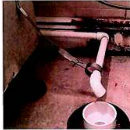
Residential Area Ice Machine Drain Line
