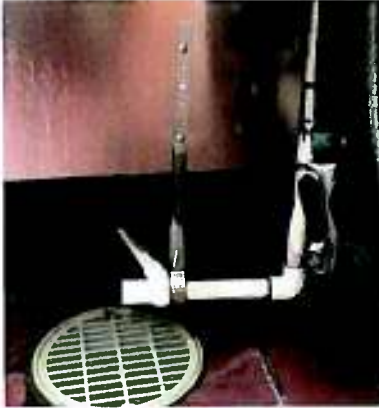
Kitchen Ice Machine Drain Line
