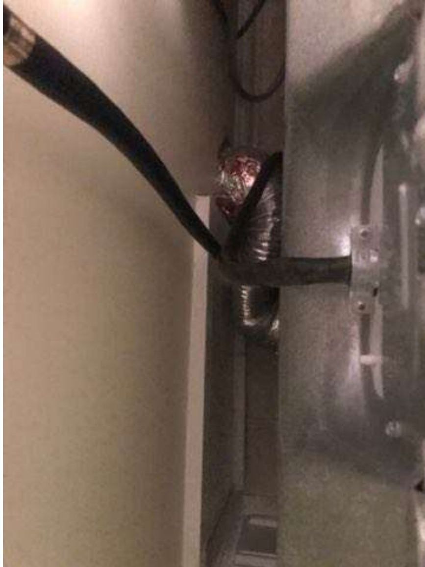
Behind the dryer view
