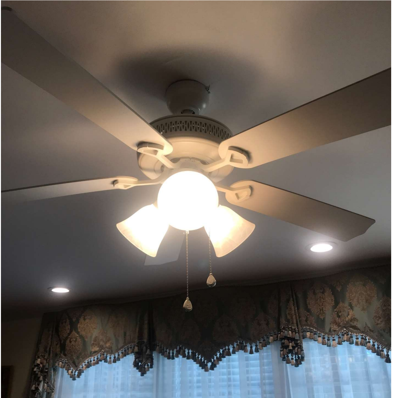
Light fixture in the Dining Room (all sockets have light bulbs and working properly)
