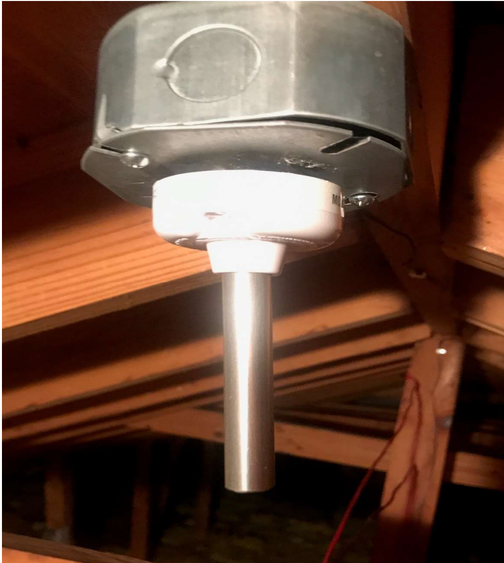
Attic Heat Detector securely mounted
